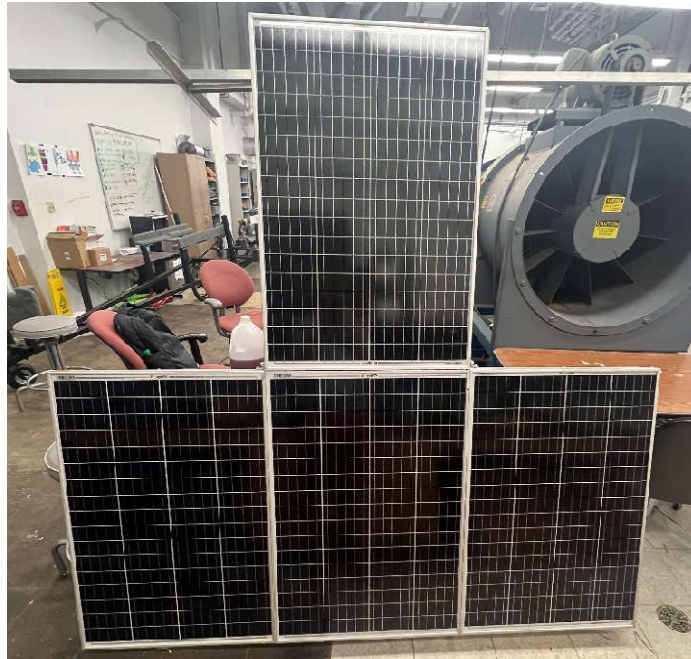
Fig. 1. Current Solar Panel Arrangement
